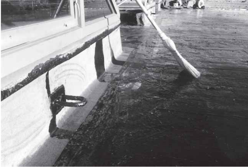
◀ The RedLINE expansion joint installed along the roof skylight. Note the cold applied modified bitumen flashing.
