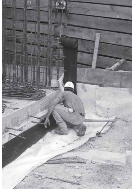
▲ The FlamLINE roll being unrolled and partially completed installation ready for stripping on the opposite selvage edge.
