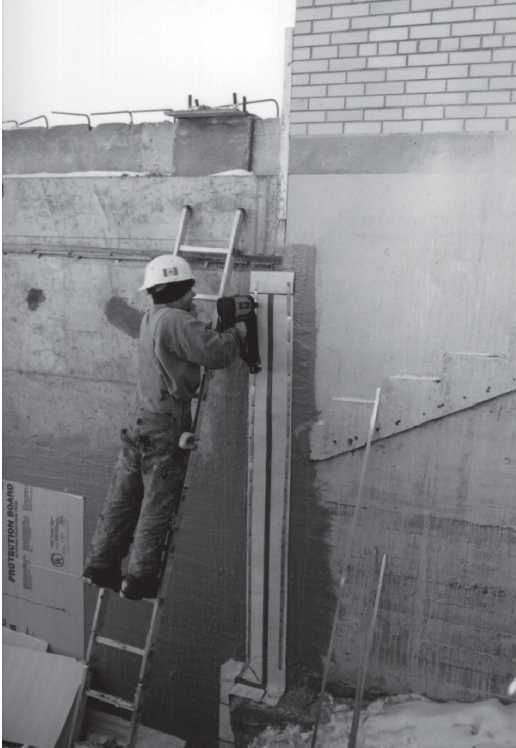
▲ The RedLINE is secured to the concrete substrate with termination bars all the throughout its height.
