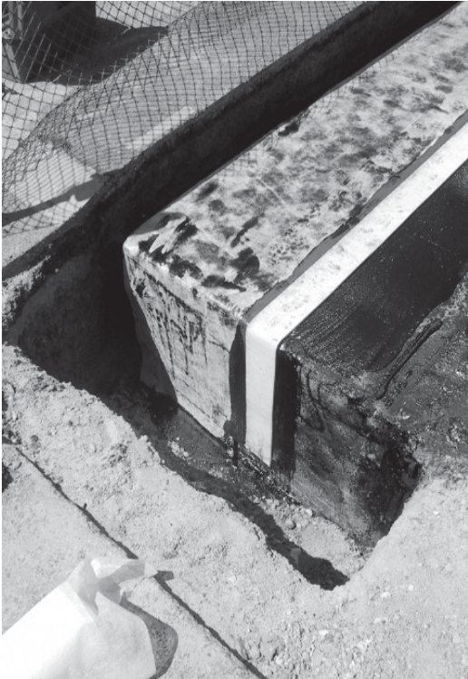
▲ Reinforcing fabric applied to one side of the RedLINE joint (joint termination shown).
