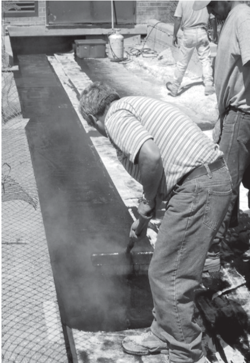
▲ Applying the second coat of hot rubberized asphalt over the reinforcing fabric.
