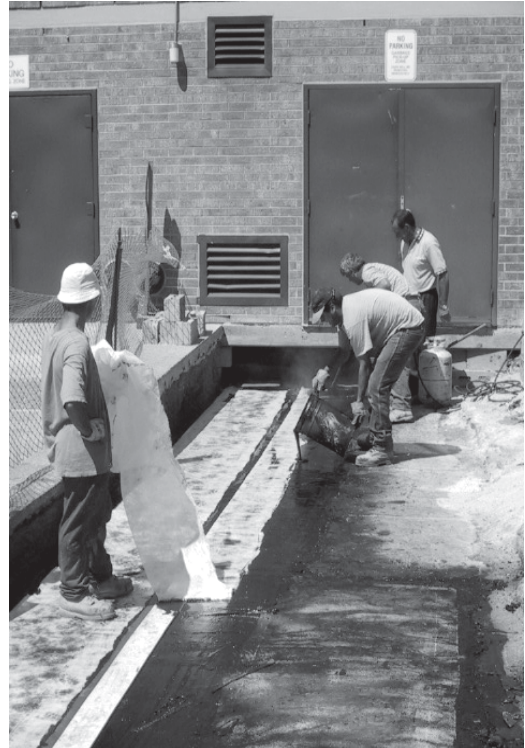
▲ Applying the HRA reinforcing fabric on to the RedLINE as per the hot rubber manufacturer requirements.
