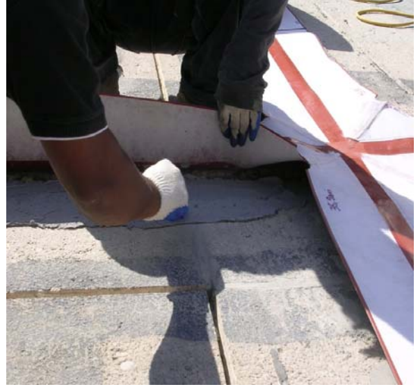
Epoxy is being applied to the substrate to adhere the RedLINE joint
