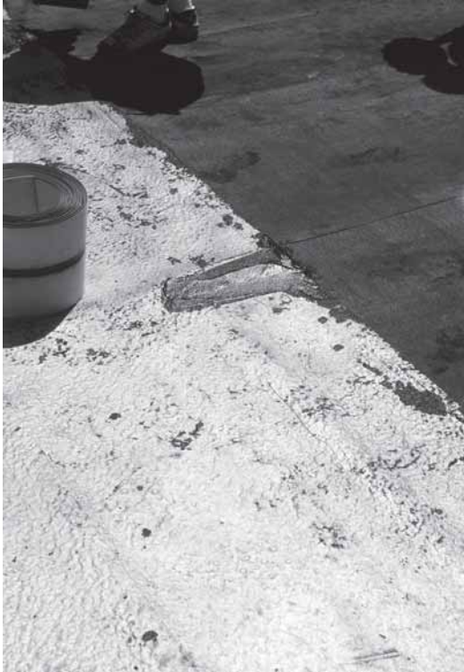
▲ The expansion joint is identified on site and the RedLINE is checked for proper fit.
