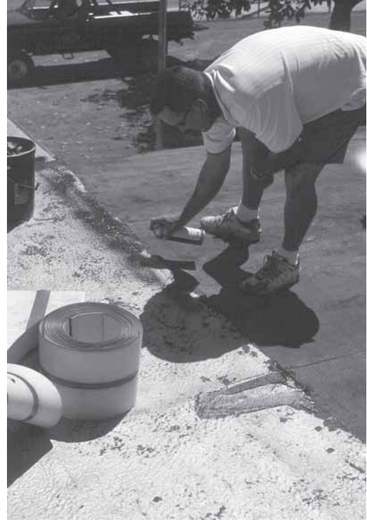
▲ Prior to the application of the RedLINE the surface needs to be primed.
