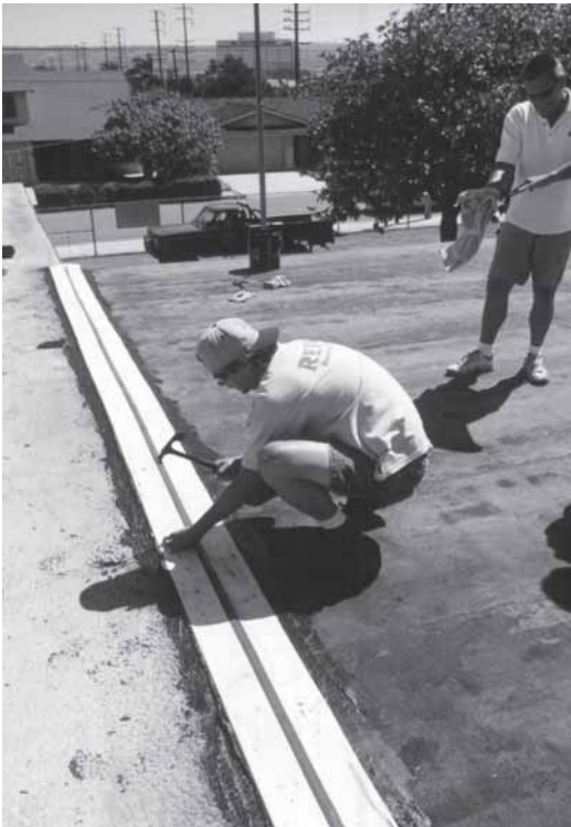
▼ The RedLINE is secured in place using flat headed nail. This necessary for temporary fixation.
