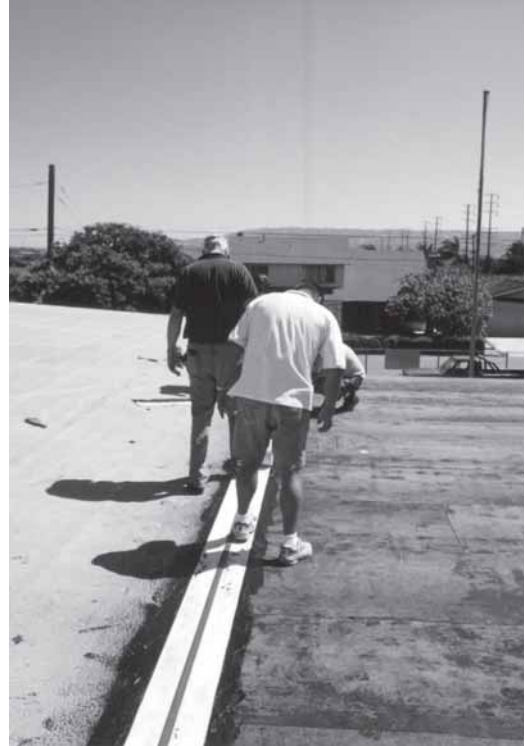
▲ Pressure is applied over the RedLINE so the fleece is fully coated with the adhesive.
