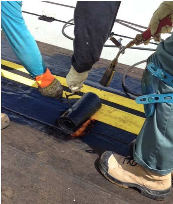
Base flashing is being torched half way onto the yellow selvage edge.
