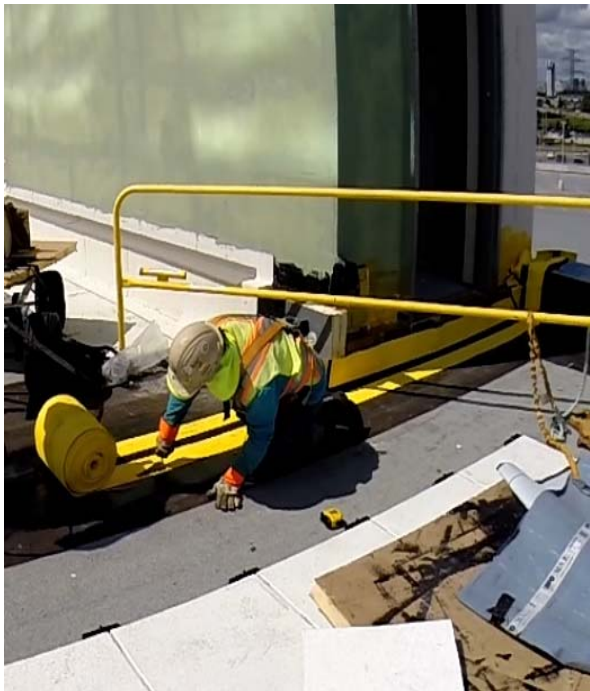
Pressure is applied to the FlamLINE to ensure proper adhesion and bleed out.
